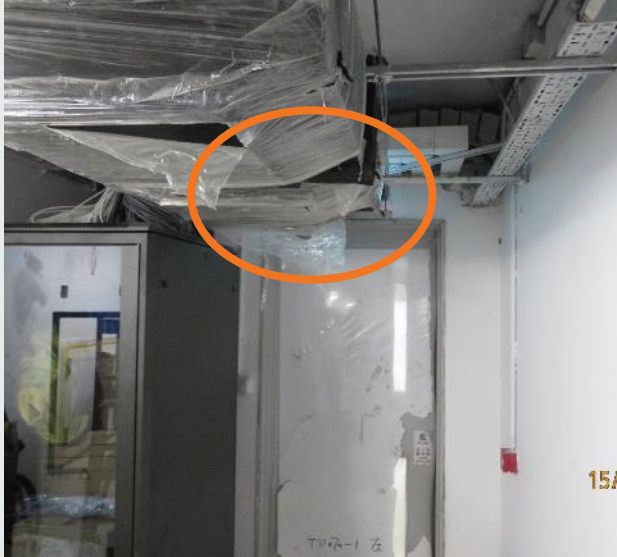
Exit Sign was obstructed by vent duct
