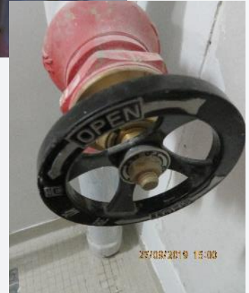
Hand-wheel's operation ineffective
