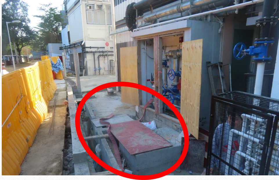
Sprinkler inlet & Control Valve Group were inaccessible
