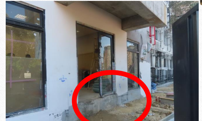
Improper Means of escape
