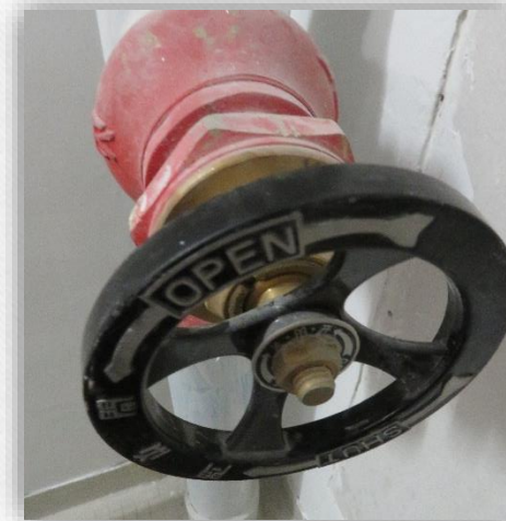
Hand-wheel's operation ineffective
