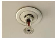
Automatic Sprinkler System
