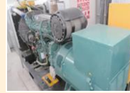
Secondary Source of Electrical Power Supply
