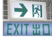
Exit Signs (including Directional Signs)
