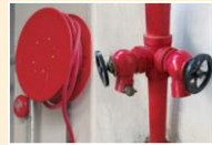
Fire Hydrant and Hose Reel System
