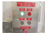
Automatic cut-off device for Mechanical Ventilating System
