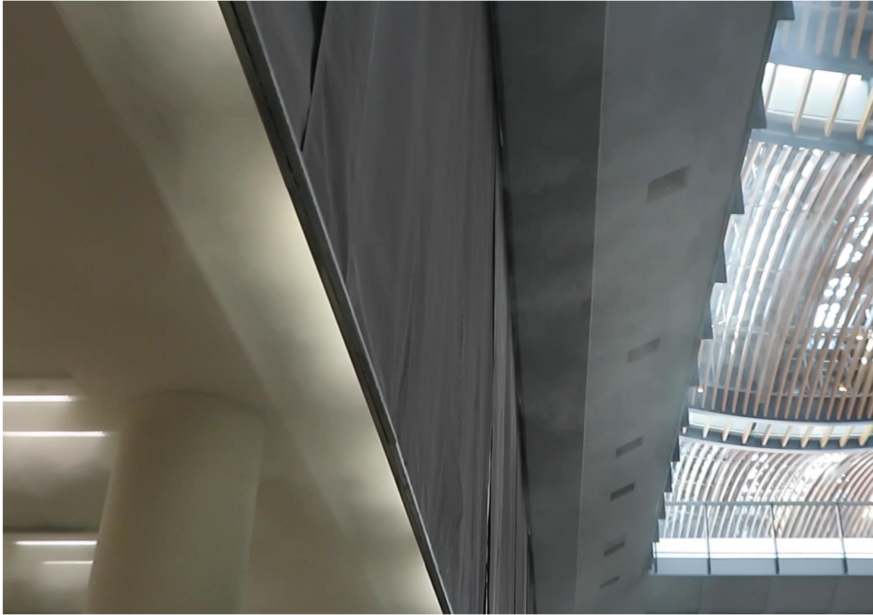
Smoke curtain failed to contain smoke ✘
