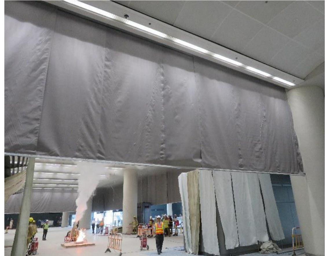
Prevention of smoke spread by smoke curtain
