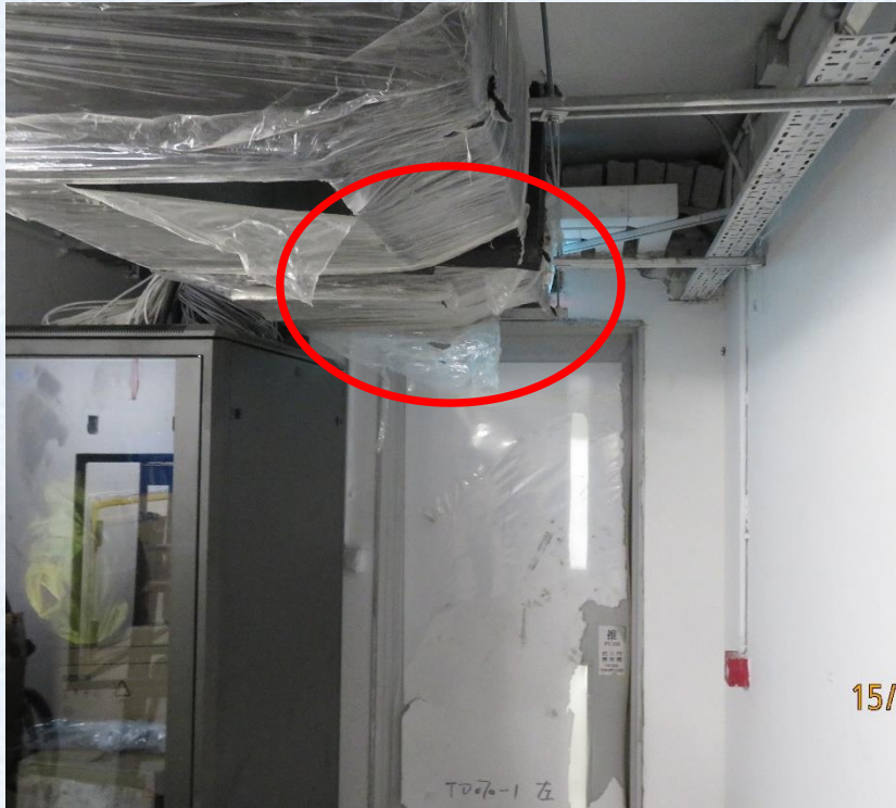
Exit Sign was obstructed by vent duct
