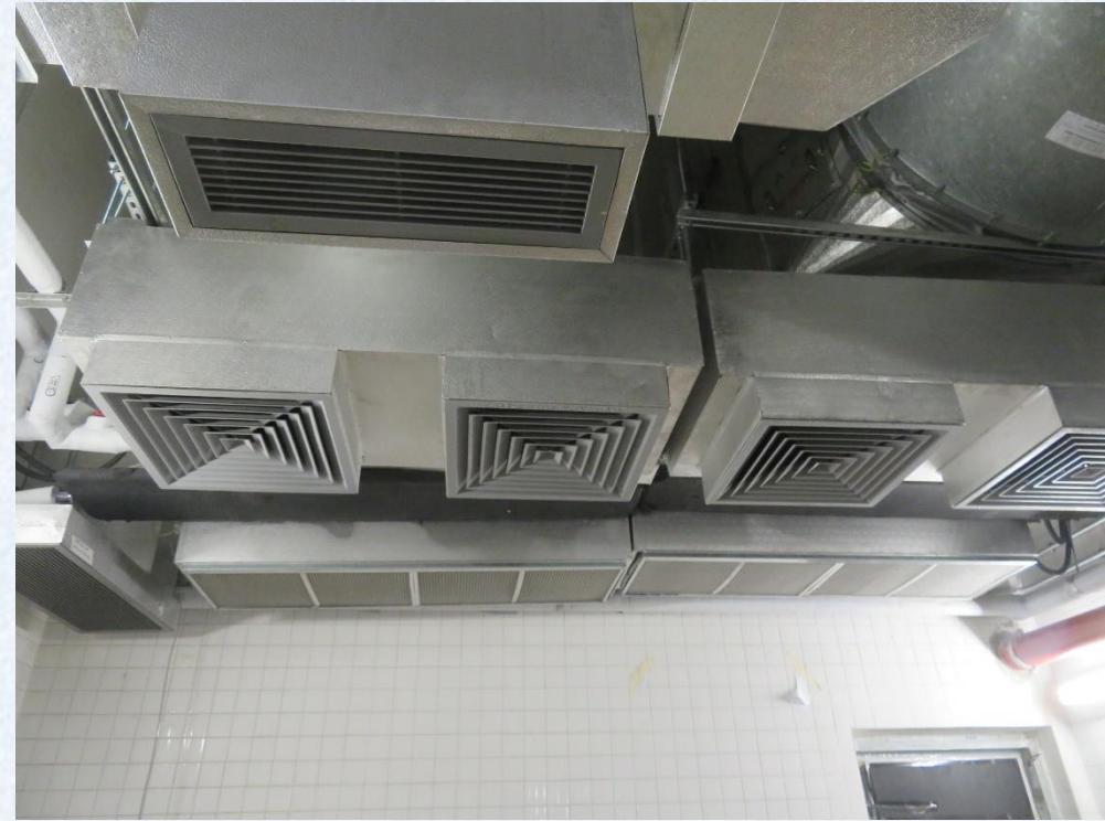
Sprinkler heads were obstructed by ductworks
