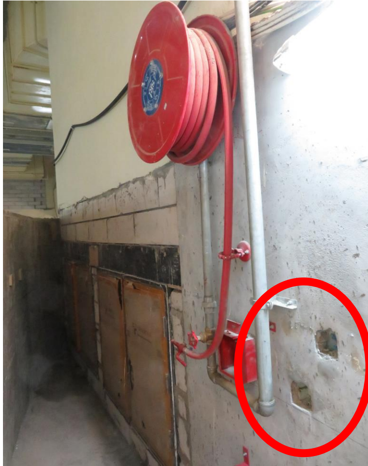
Missing of Break-glass Unit for FH/HR System
