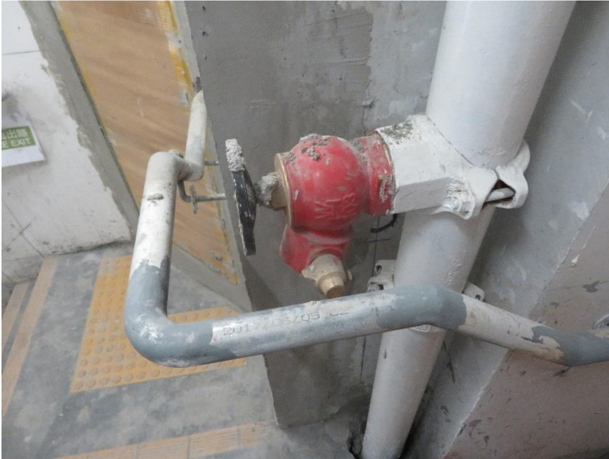
Fire hydrant / hose reel obstructed by building structure
