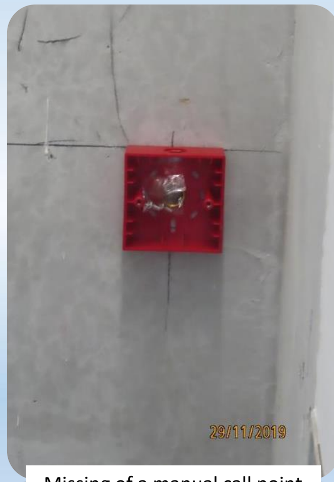
Missing of a manual call point
