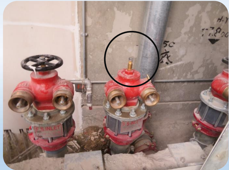
Center of coupling more than 1000 mm above ground level
