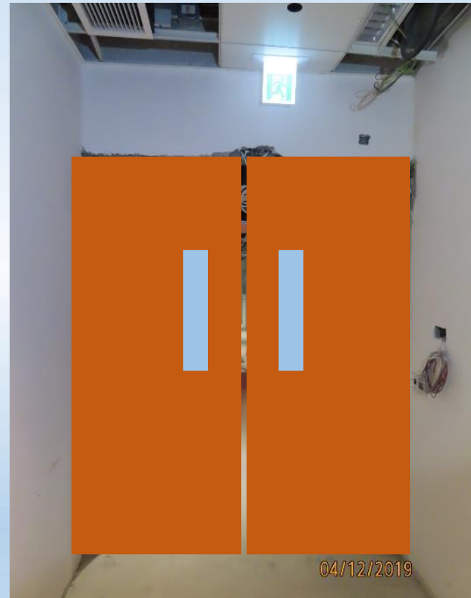
Smoke Stop Door found missing
