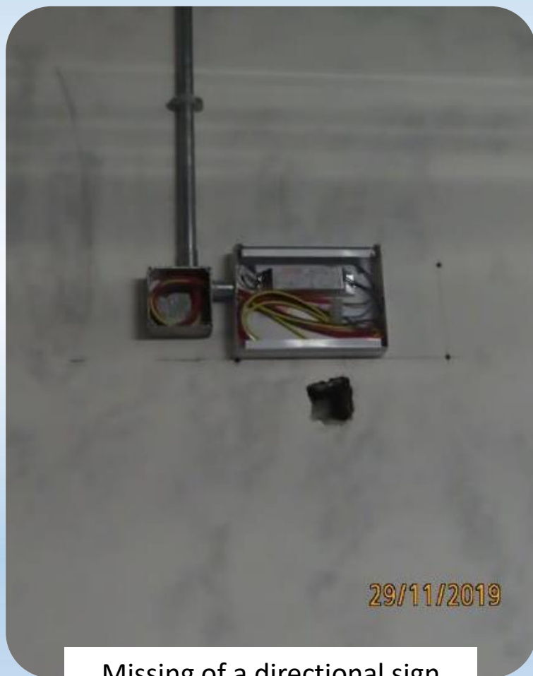
Missing of a directional sign
