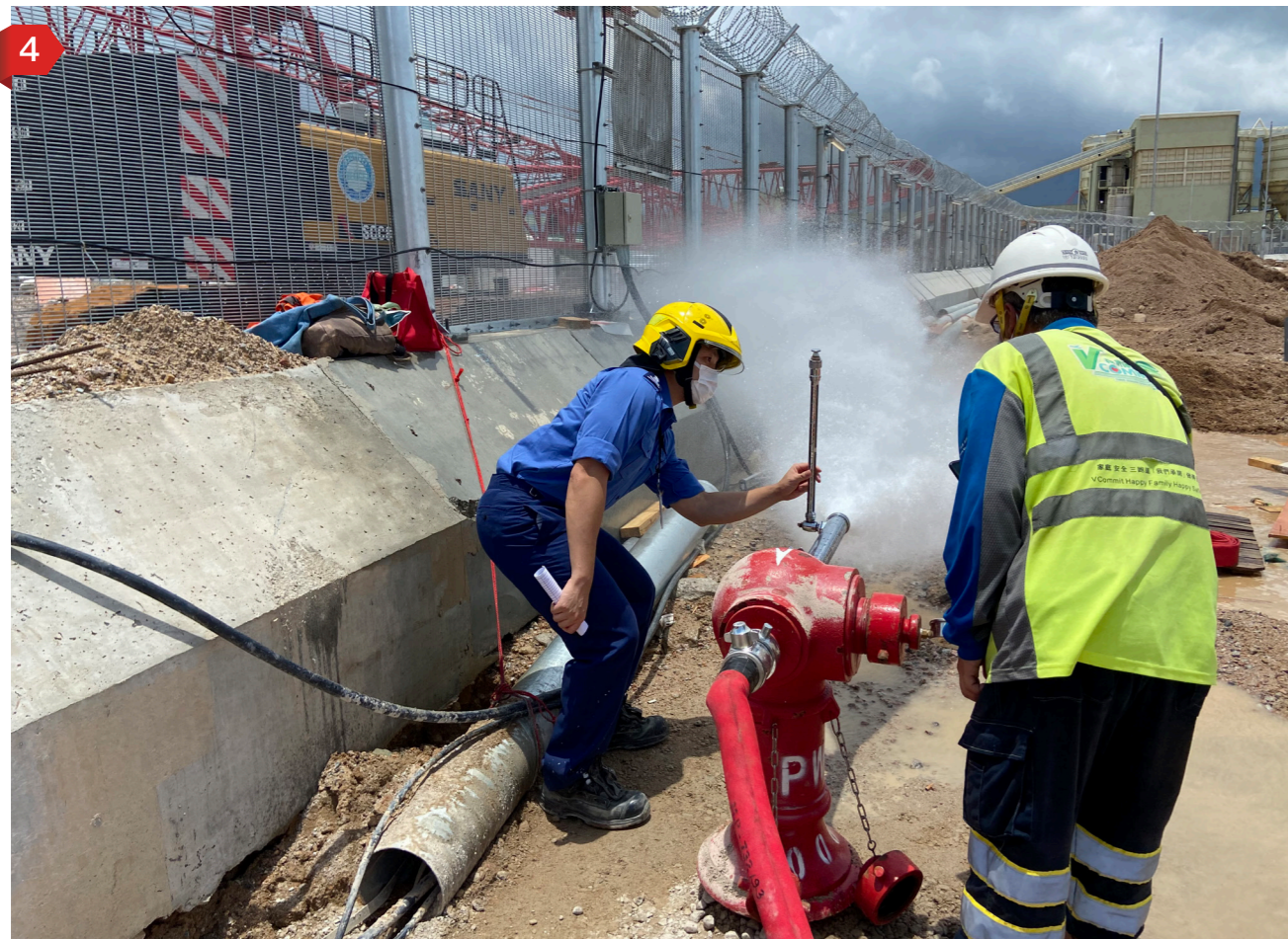
4 機場擴建工程課人員正驗收三跑道系統的消防柱。 Airport Expansion Project Division personnel is conducting acceptance inspection for a street fire hydrant of the Three-Runway System.
