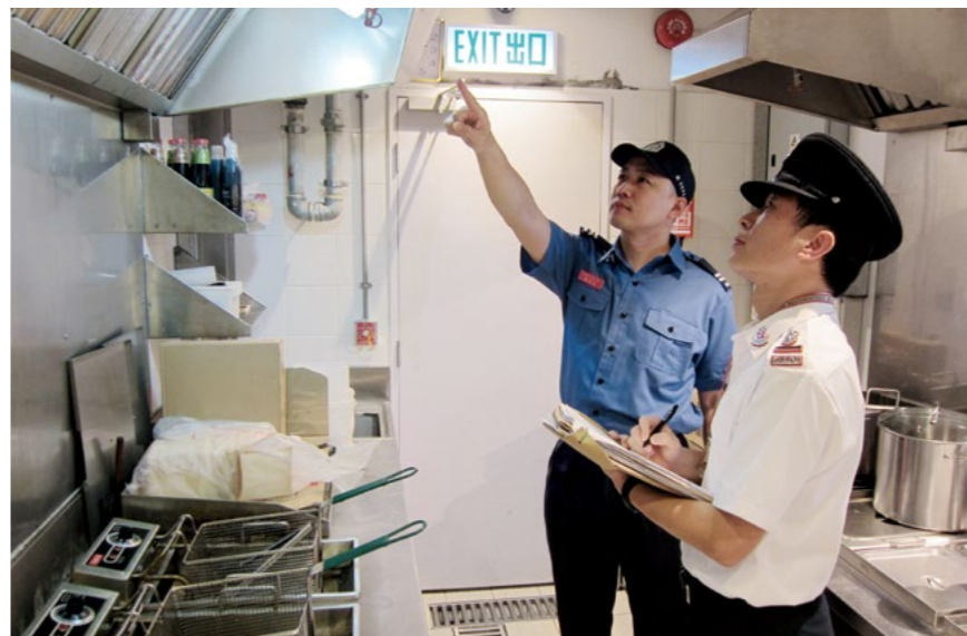
c. 消防人员到食肆巡查,确保其消防装置及设备合乎消防规定。 Fire personnel inspect a food premises to ensure that its FSIs and equipment are in compliance with the fire services requirements.
