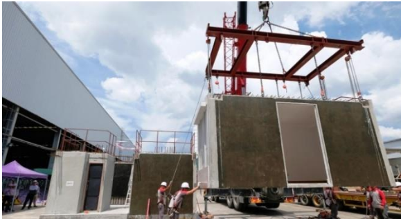
The adoption of MiC to the construction of Fire Services Department Pak Shing Kok Married Quarters
