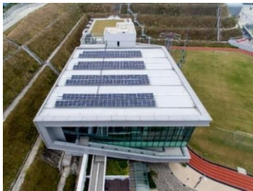
The PV panels installed at Physical Training Complex at Fire and Ambulance Services Academy
