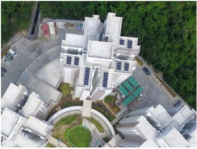
The photovoltaic panels installed in the quarters
