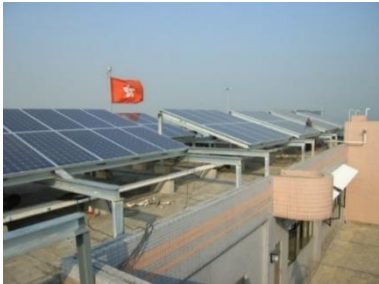
The PV panels installed at Chek Lap Kok Fire Station
